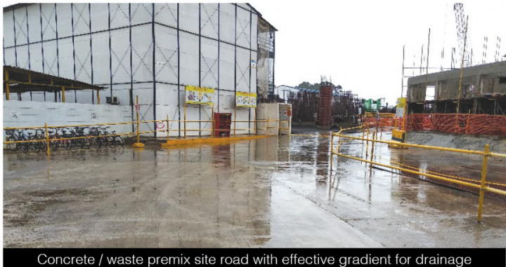
Concrete / waste premix site road with effective gradient for drainage
